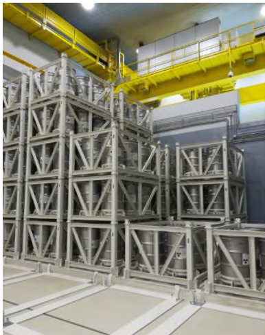
New low level radioactive waste Interim Storage in Latina – Italy [26]
