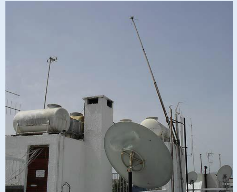
FIG. Example of a deteriorated structure with an RLC. Courtesy of the Department of Labour Inspection, Cyprus.
