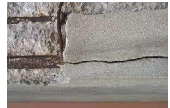
Rebars corrosion and mechanical damage on concrete
