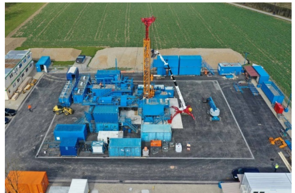
Drone photo of the drilling site in Bülach after setting up the drilling rig ( www.nagra.ch )
