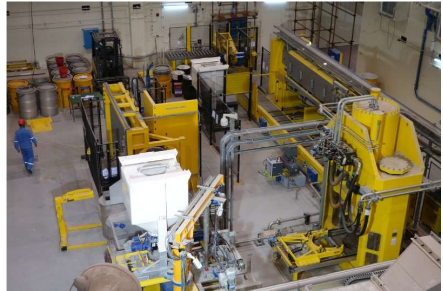
Facility for storage, compacting and cementing radioactive waste, Source: Bilfinger .
