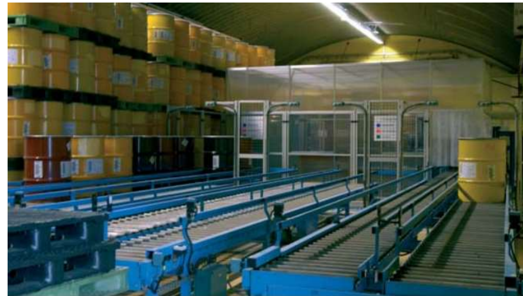
Storage hall for waste drums after characterization on automated lines at Saclay. Source: CEA (France), 2006 Report
